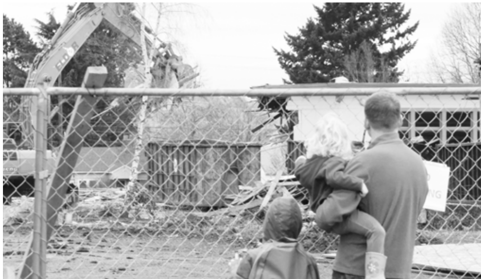
An excavator with a demolition bucket drops its mouthful of the old Faubion School into a dumpster. Photo by Carl Jameson
